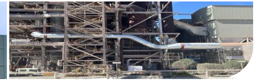
Hydrogen calcination pilot Construction is underway at Yarwun for this world first technology
