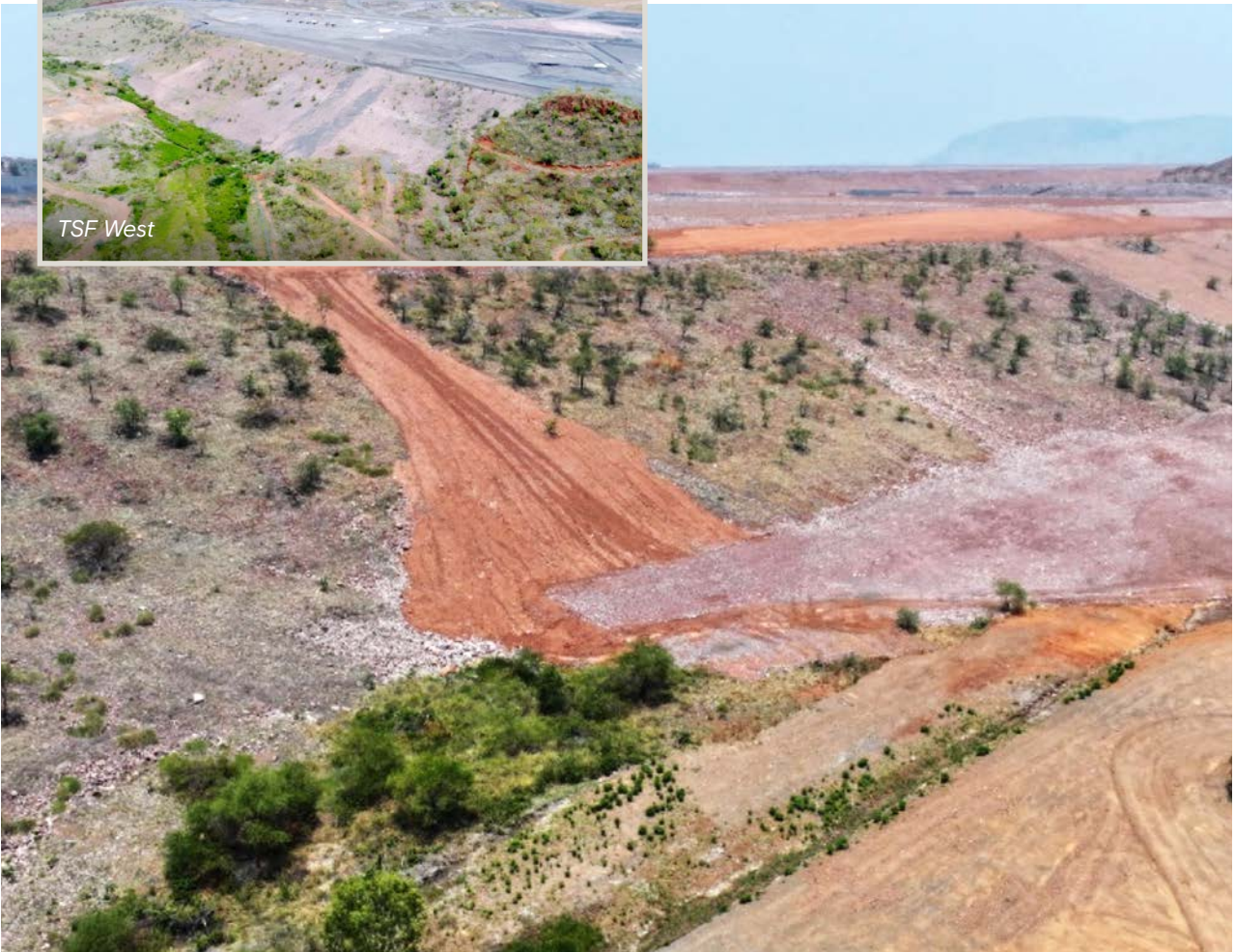
TSF West Retention Paddocks, Dam Embankment and Light Industrial Area (LIA) Embankment completed
