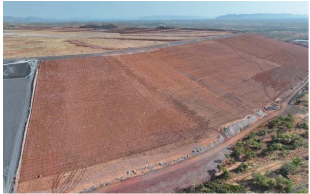
Ongoing growth media spreading and ripping on the TSF main dam embankment
