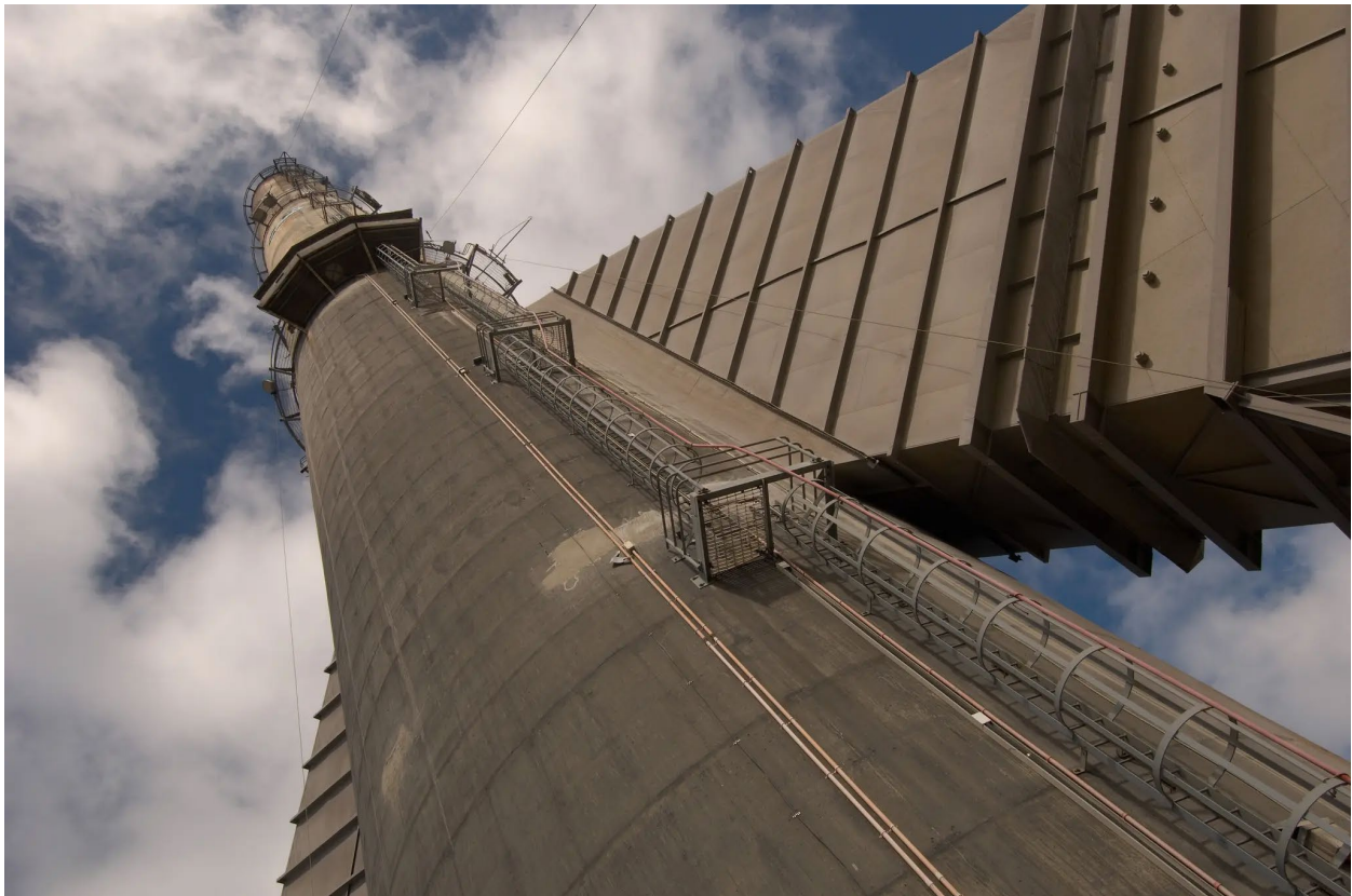
NZAS main stack
