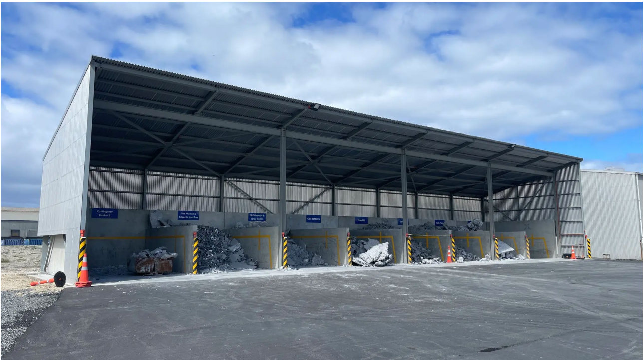
NZAS waste segregation area
